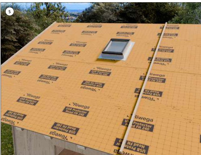
5 After laying the membrane on the roof pitch without folds, secure it with a second counter-batten
