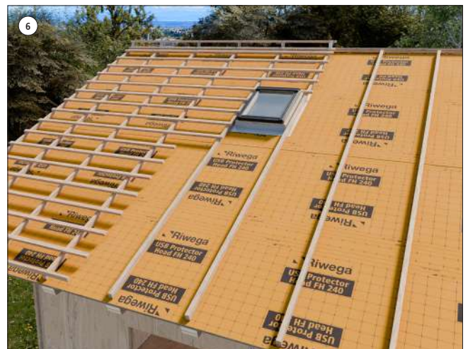
6 Finally, proceed with the placement of the remaining counter-battens and roof tile holder slats
