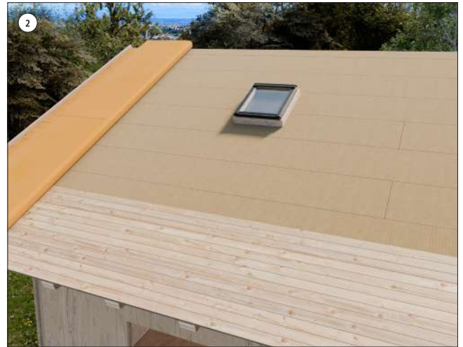
2 Unfold the membrane starting vertically and attach the first counter-batten to the edge of the pitch
