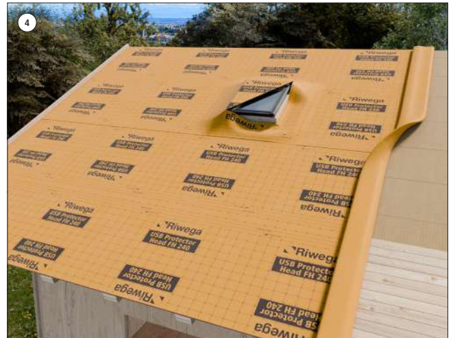
4 Cut the membrane and seal it around the parts emerging using the appropriate accessories
