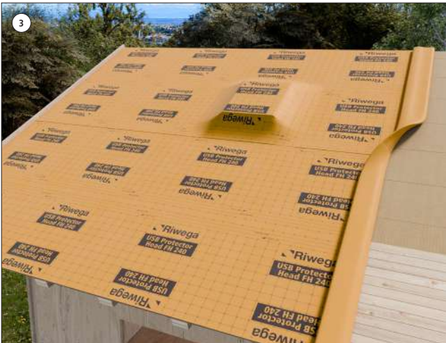
3 After securing the counter-batten on the edge, unfold the membrane by proceeding horizontally
