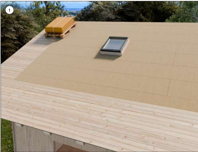
1 Place the pallet containing the folded membrane on top of the pitch to be covered
